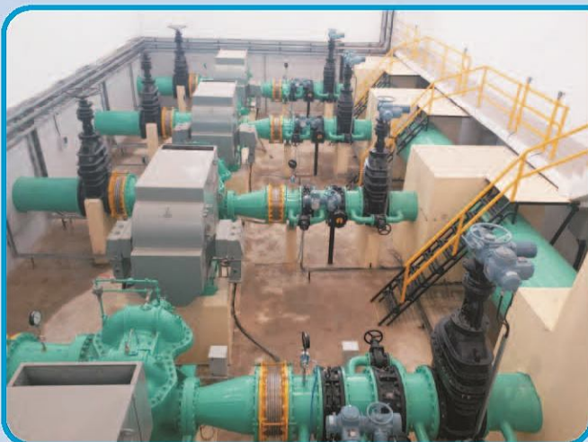
Navda SPP 3B Pumping Station
